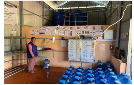
Figure 22: Water Kiosk (Owe) operation run by a woman entrepreneur in Tuek
